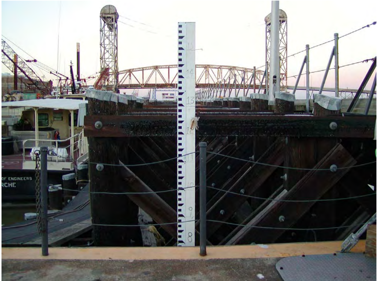
Figure 1-57. Staff gage at IHNC lock. Numbers were far more visible when the lock was visited in October 2005. Picture looking north.
