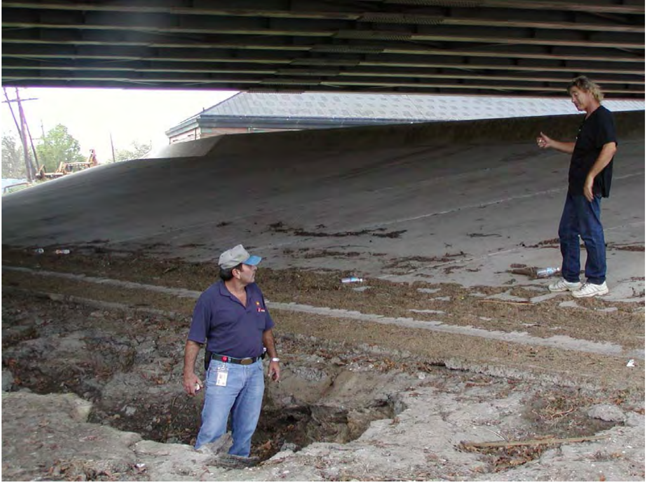
Figure 1-77. Scour below concrete apron that is below low pump station wall on east side of Orleans Ave Canal.
