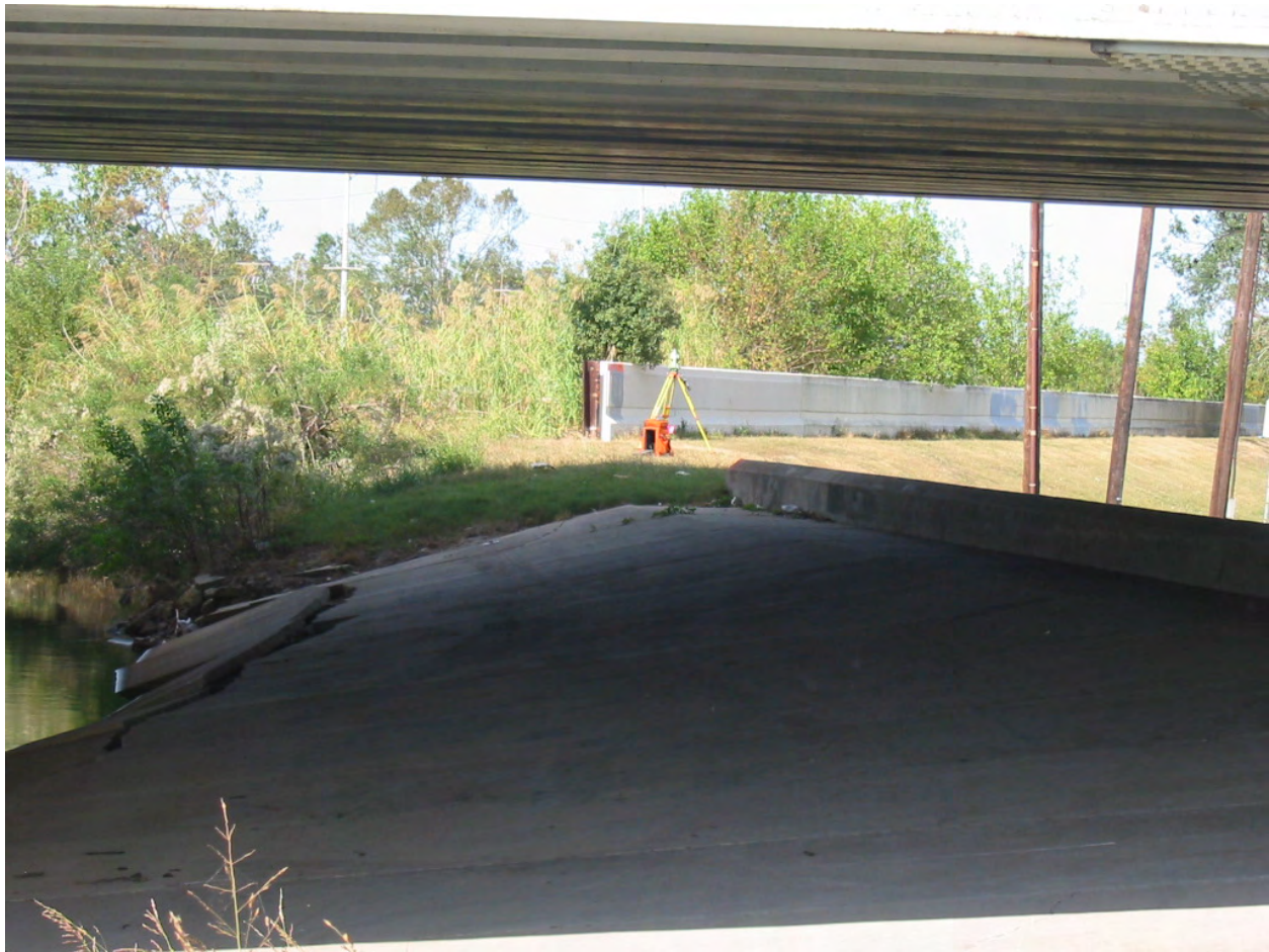
Figure 1-72. Low wall, earth levee, and floodwall in background on east side of Orleans Avenue Canal just north of pump station. Looking northwest.
