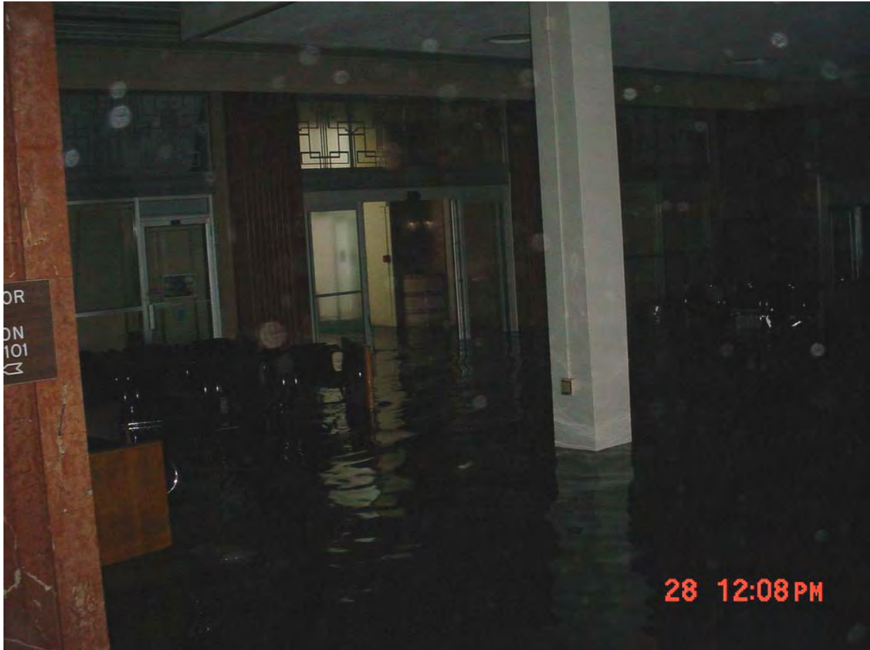
Figure 1-48. Time = 12:08, APH-09. On column in terminal building lobby.
