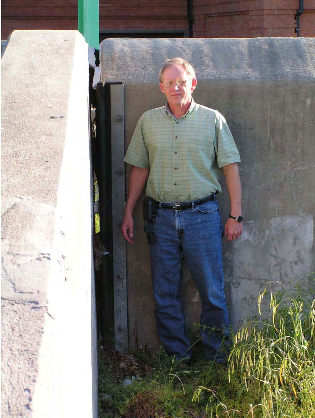
Figure 1-86. LA 1251 at crack in wall. Picture taken 4/06/06. Debris in crack was 2.2 ft below top of wall on 9/29/05.
