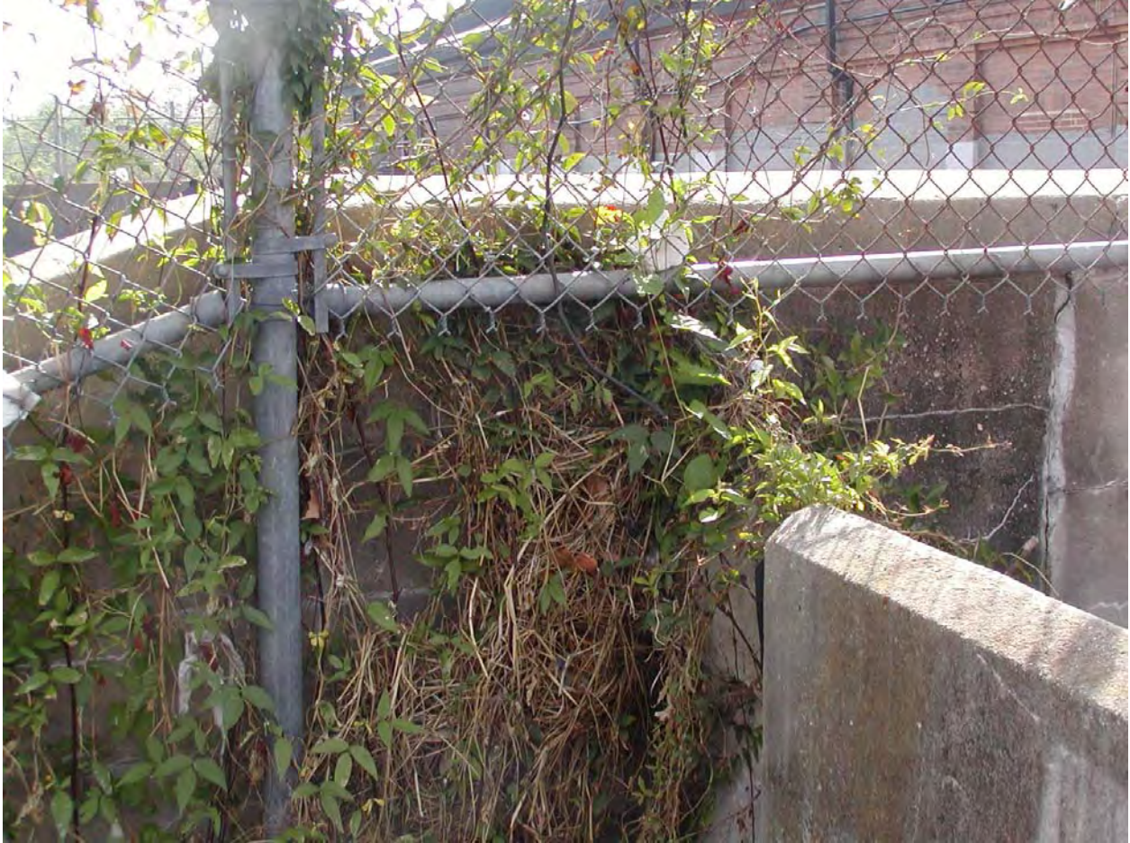
Figure 1-79. Debris caught in vegetation showing flow over low wall at OP#7. About 6" above low wall on west side.
