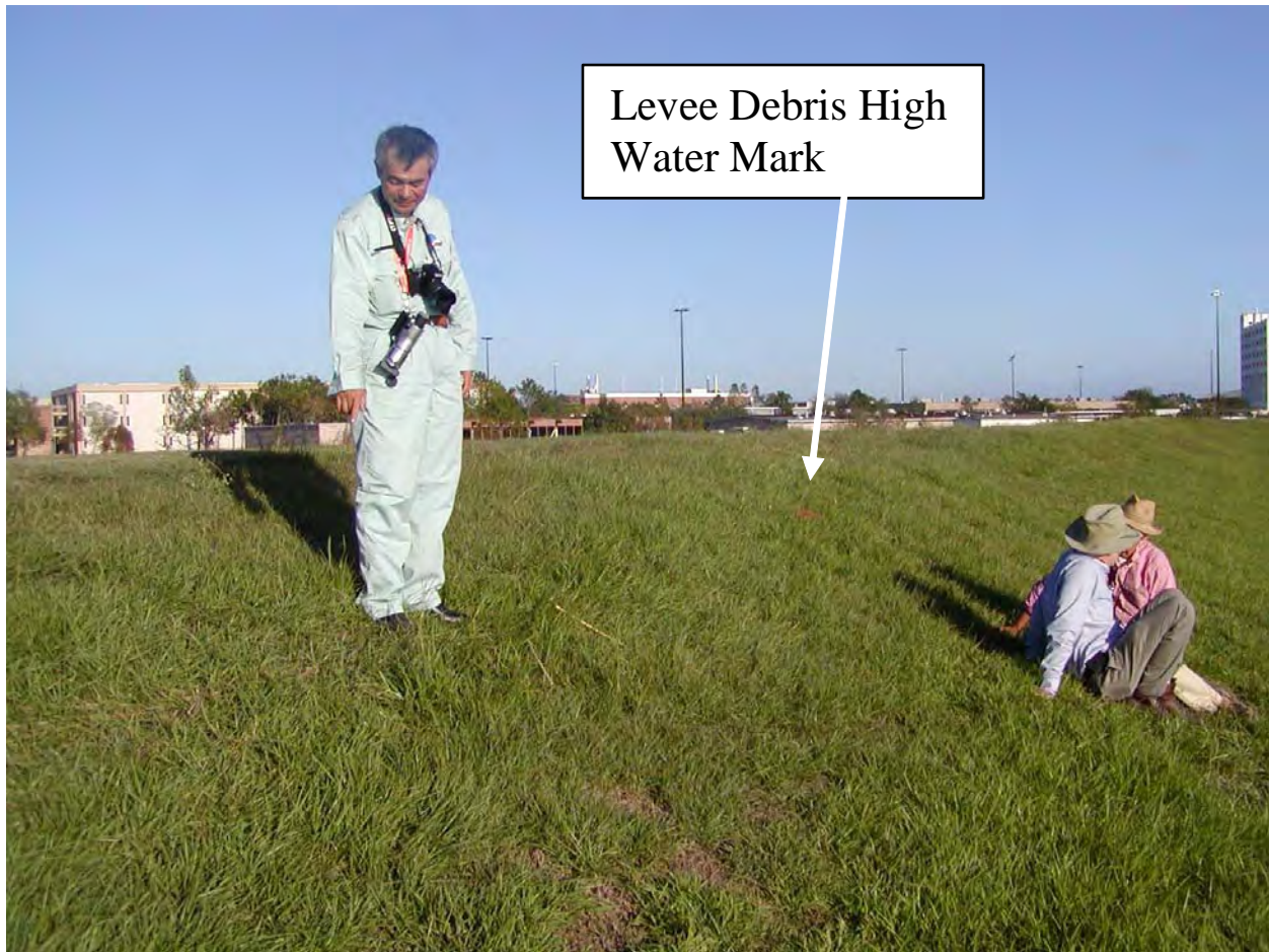
Figure 1-96. Debris high water mark LA 1022 on east levee of London Avenue Canal north of Leon C Simon Drive.
