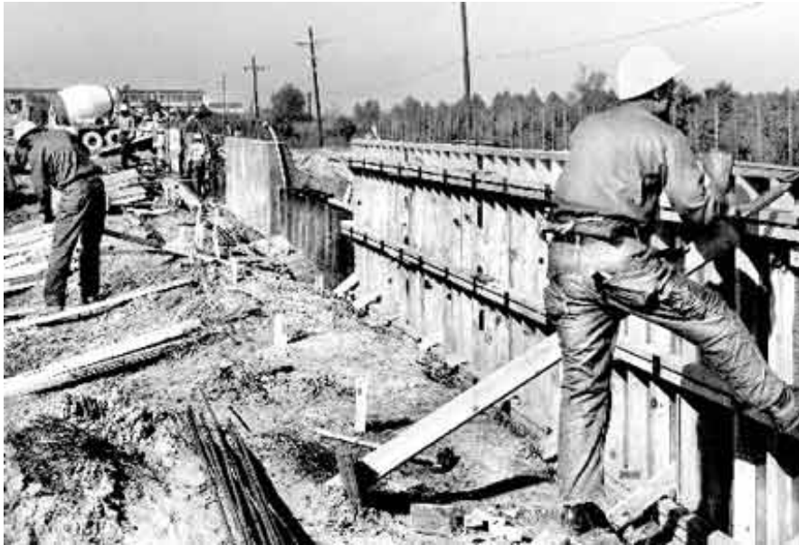
LEVEE-BUILDING IN 1968 - Three years after Hurricane Betsy, the Army Corps of Engineers began building the first concrete floodwalls along the east bank of the Inner Harbor Navigation Canal. Here, the floodwalls between Hayne Boulevard and Dwyer Road are built by placing concrete over steel pilings that were driven into existing levees earlier in 1968. (Staff file photo)
