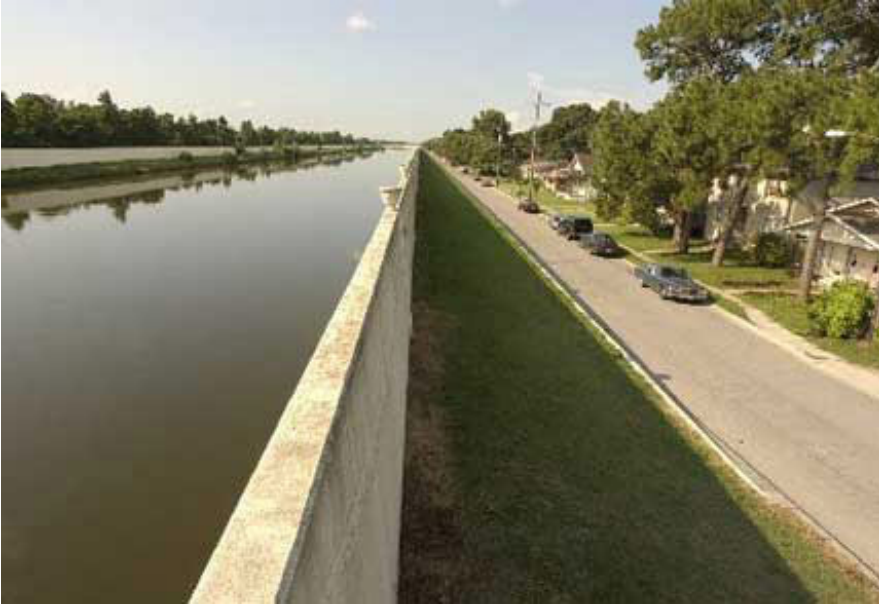
WATER ALL AROUND US: BARRIER LINES - A floodwall divides Orleans Avenue from the Orleans Avenue Outfall Canal, one of the many drainage canals that channel storm water into Lake Pontchartrain. In a catastrophic storm, the lake would back up into the canals, giving the floodwaters a beeline straight into the heart of the city. (PHOTO BY ELLIS LUCIA / The Times-Picayune)
