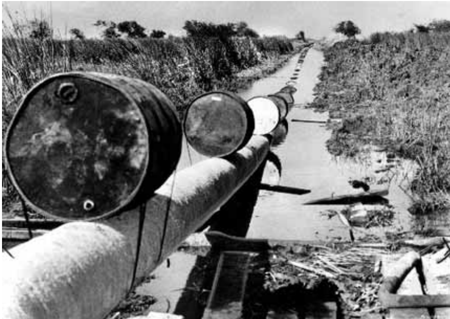
Oil pipelines coated in concrete buried throughout south Louisiana. But today, many lie exposed in marshes where once-sold land has eroded around them.
