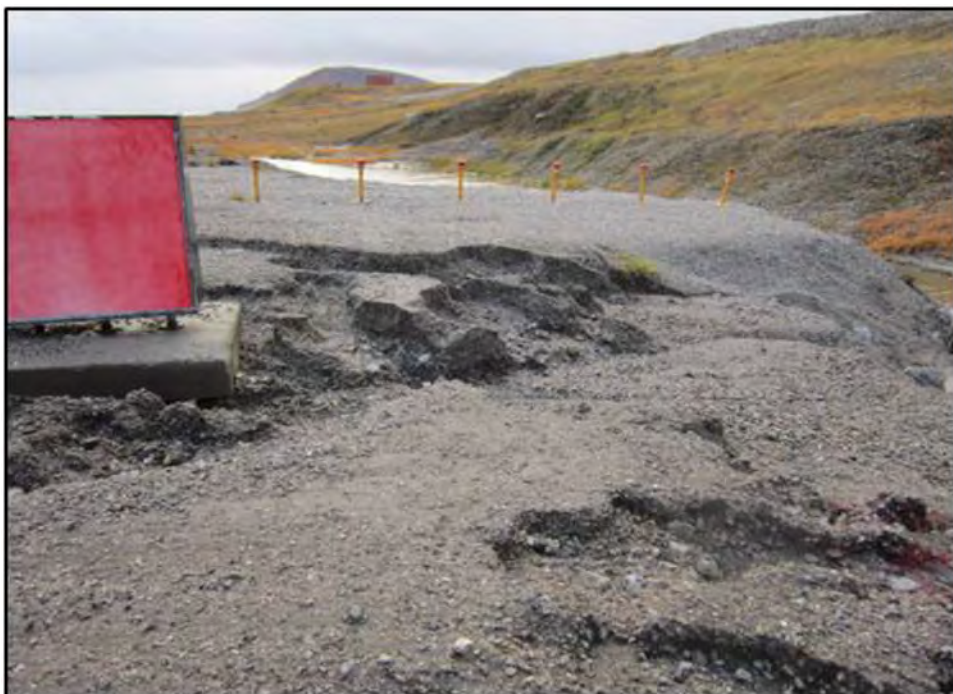
Figure 1: Overrun area of Air Force runway impacted by erosion
