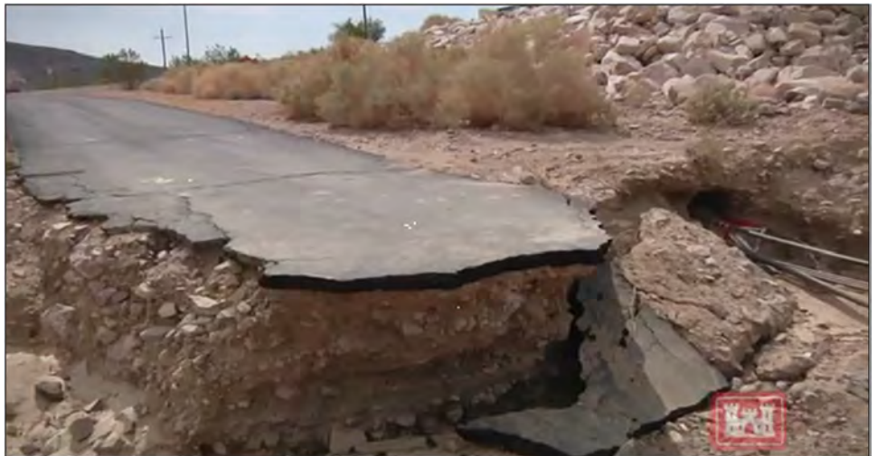
Figure 8: Video Still Showing Damage to Infrastructure at Installation located in Southwestern United States
