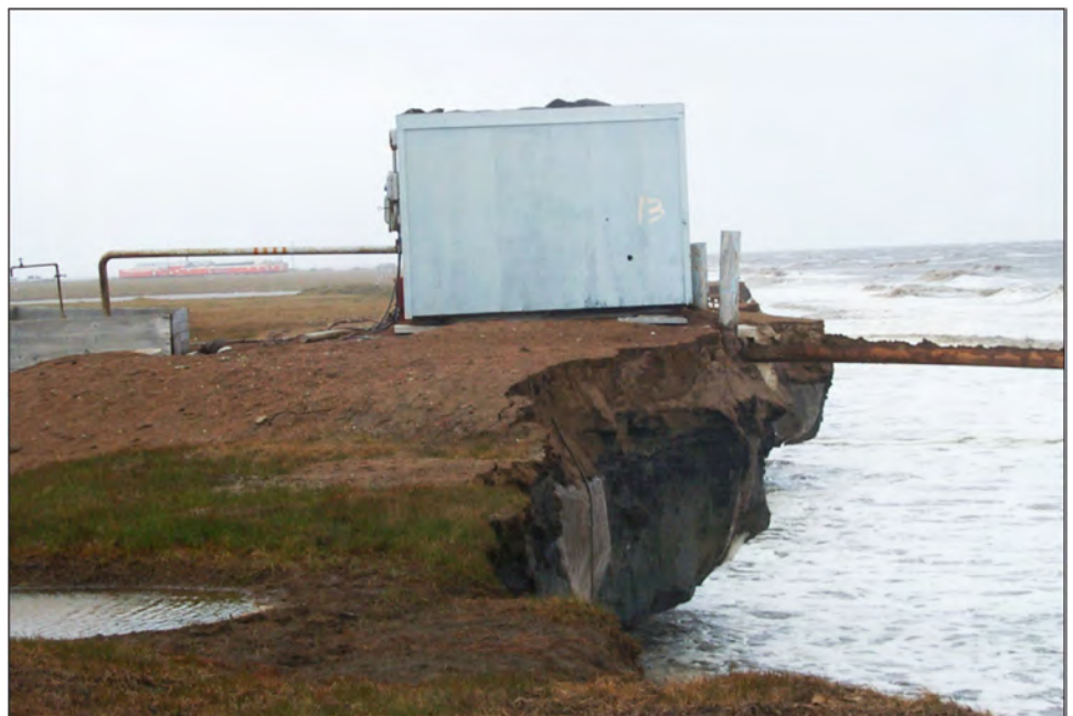
Figure 7: Coastal Erosion near DOD Early Warning Site
