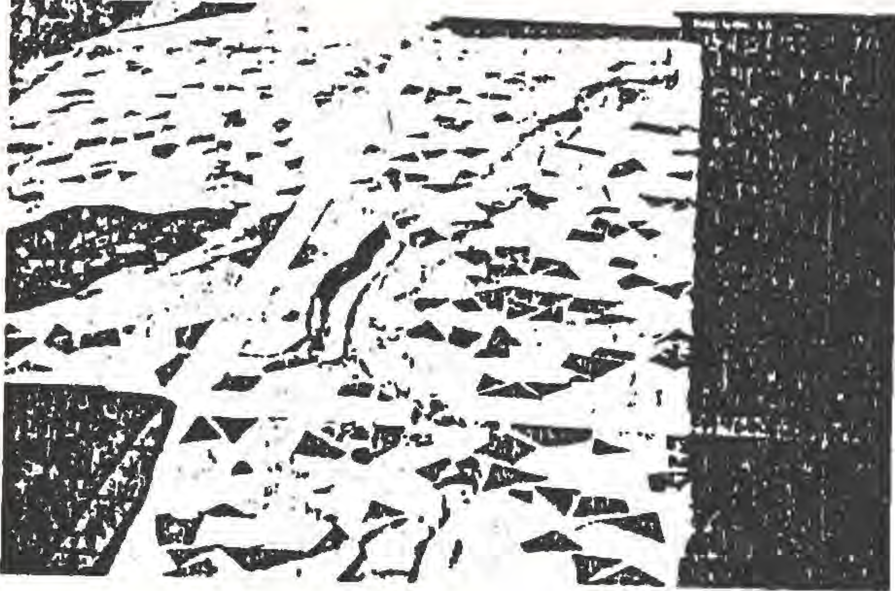
PAVEMENT CRACKS - 5115 Crown (fault associated)
