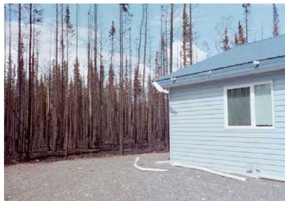
Tok, AK. . This house survived a wildfire almost untouched due to the defensible space surrounding the structure and the use of metal siding and roofing. The only visible damage is to the plastic rain gutters, which softened due to the heat and fell to the ground. Image courtesy of Alaska Visitor Information Services.
