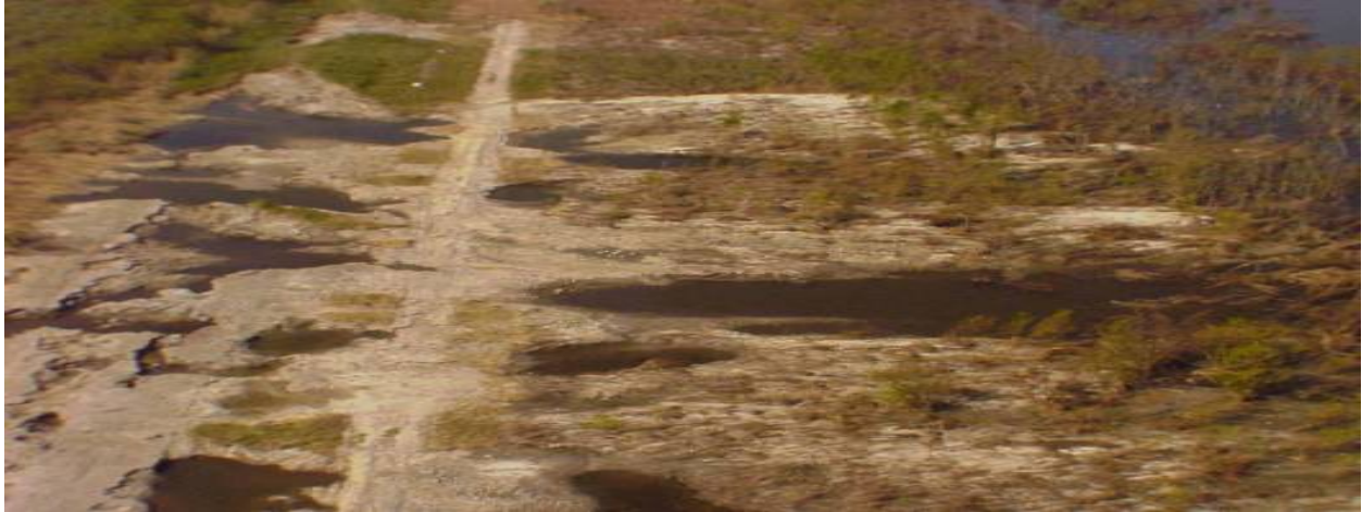
Figure 19. Example of levee along New Orleans East, GIWW, breaching from overtopping and scour of erodible materials.
