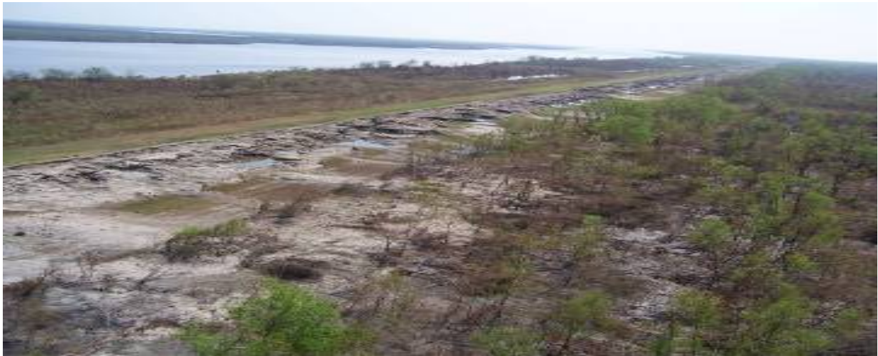
Figure 20. Example of levee breach along MRGO from overtopping and scour of erodible materials.
