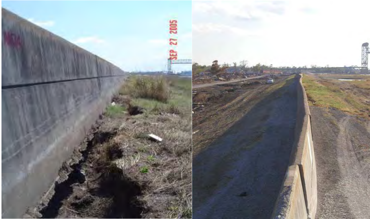
Figure 49. IHNC East Bank – North Breach – Wall Movement
