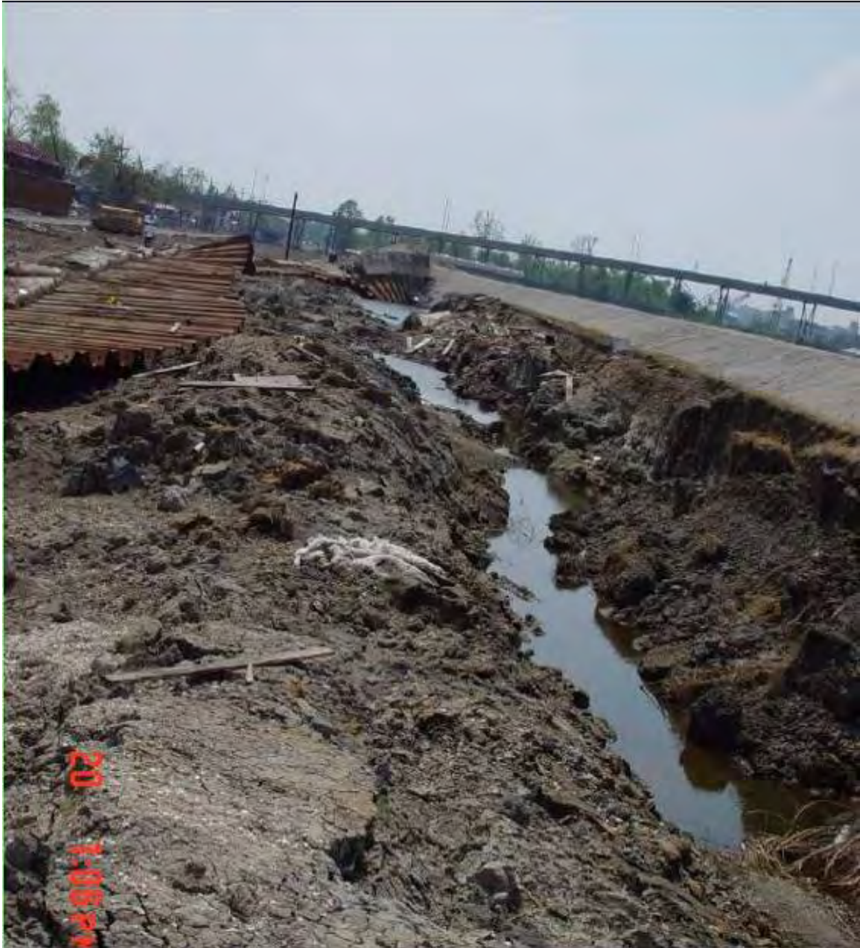
Figure 46. Scour and Erosion Leading to the Failure of the I-Wall on the IHNC Adjacent the South Breach (9th Ward)
